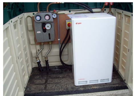
NEAT GSHP INSTALLATION IN EXTERNAL CABINET
