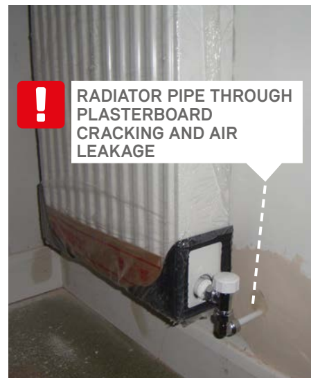
AIR LEAKAGE TO OUTSIDE AND UNDERSIZED RADIATOR
